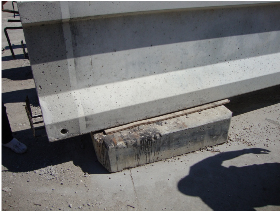
Figure A.8. Support of a Type D 60 prestressed bridge girder stored in precast plant C
